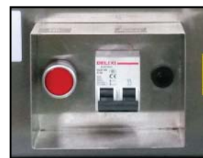
Separate "power" and "pump" controls
